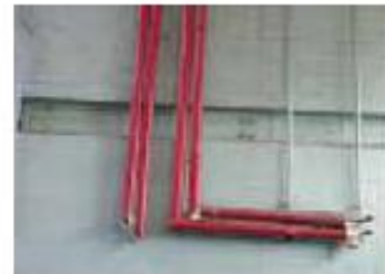
Asbestos lagging on pipes
