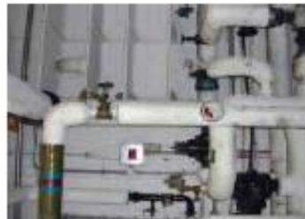
Asbestos insulation on pipes
