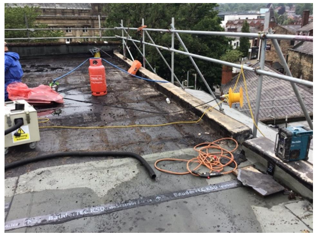
Photo 6 - Suggestion of furrings to fall from left to right in to a gutter with two chutes draining on to lower pitch roof
