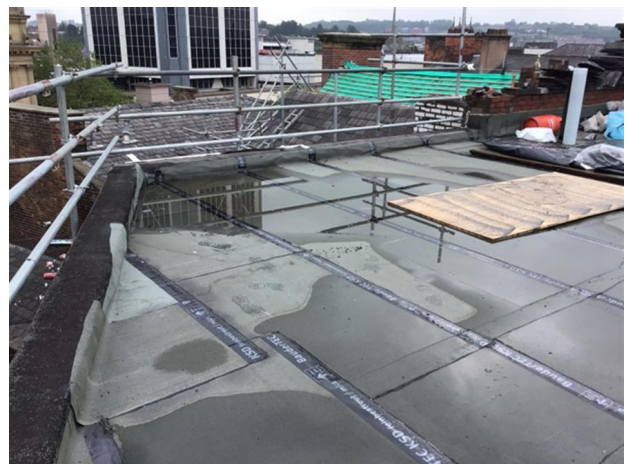
Photo 2 - View of AVCL to roof one and water in front of chute
