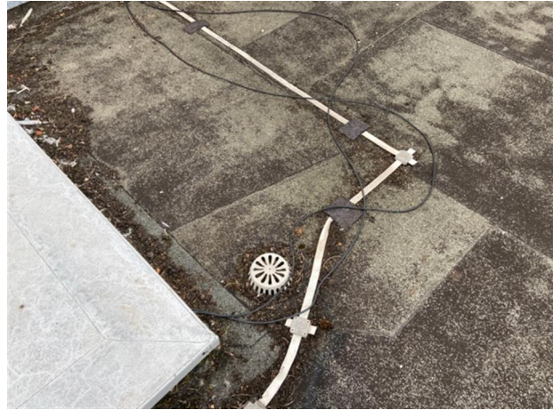
Outlet has slumped
