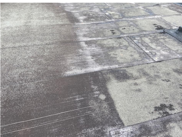
Tide marks are evident and would suggest that roof holds water
