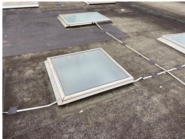
The existing wired glass rooflights will need to be changed for new fall safe units
