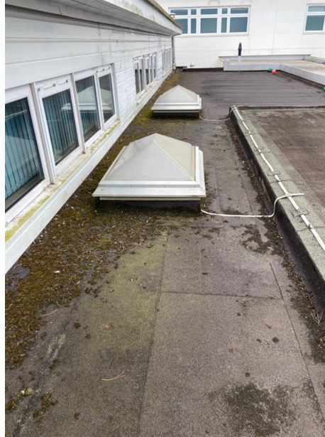
The existing felt system is starting to loose its mineral cover
