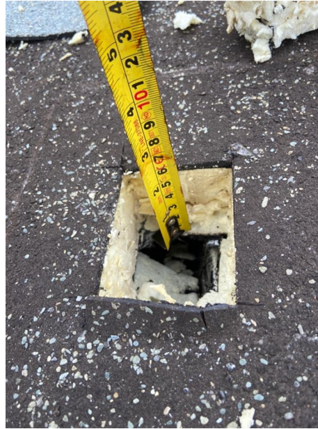
The current level of insulation falls below the 0.35 w/m2k required
