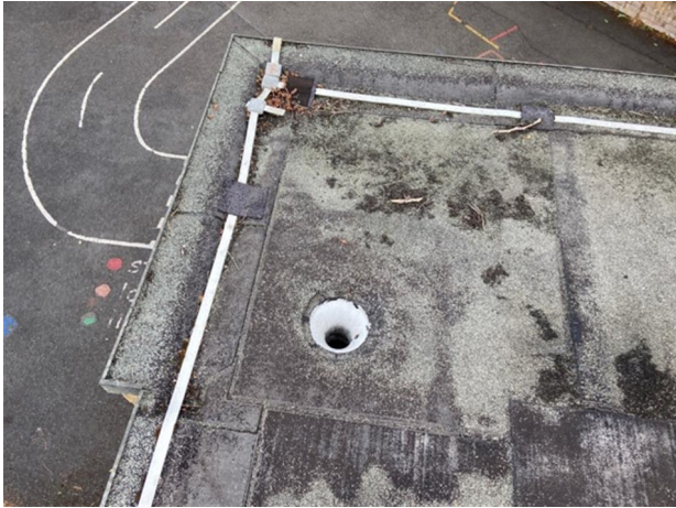
The existing outlets are old and missing leaf guards and appear to have slumped in areas
