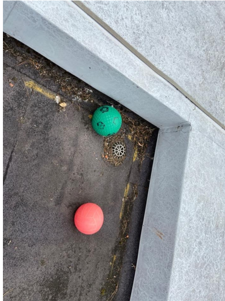
The existing outlets should be renewed with refurb outlets
