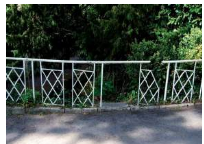
16 Canal bridges and Railway Bridges Damage to railings, signs of rust, stonework in need of cleaning.
