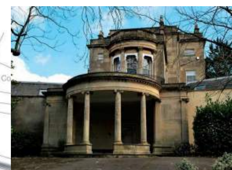
17 Loggia Stonework, interior and seating in need of redecoration and repair.
