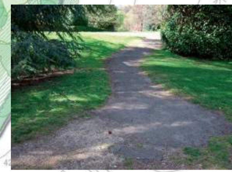
Damage to footpath surface on many paths
