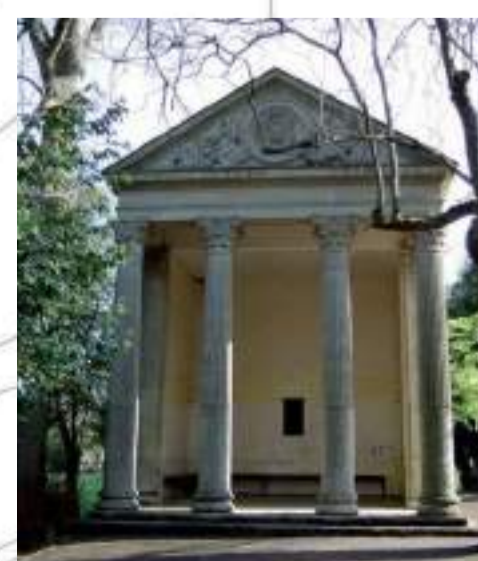
7 Minerva's temple Stonework, interior and seating in need of repair and redecoration.
