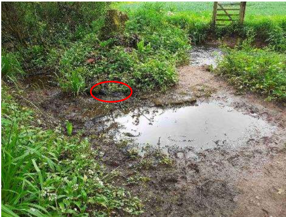
Photograph D: Foundation area on eastern bank. Land drain circled in red.
