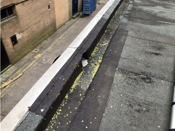
There are numerous chutes on roof area 1. A new gutter is to be formed and the chutes opened up and lined with lead.
