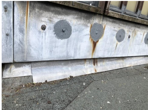
Repairs have been carried out to the lead cladding. Modification may be required to ensure that the height of 150mm can be achieved in these areas.
