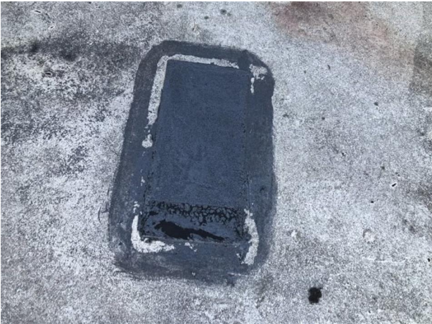
Repairs to the cracks in the asphalt on roof area 1. These will need to be removed and infilled using LiquiPaste.
