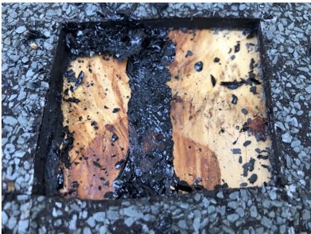
The waterproofing has been installed directly to the plywood decking with no insulation present. This will need to be upgraded.
