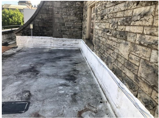
Example of the waterproofing on roof area 2. The coating is wearing away and the asphalt is slumping.
