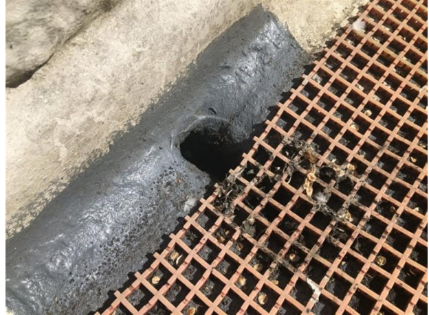
Example of one of the internal outlets on roof 2. These have no protection from debris and leaf guards are to be installed.
