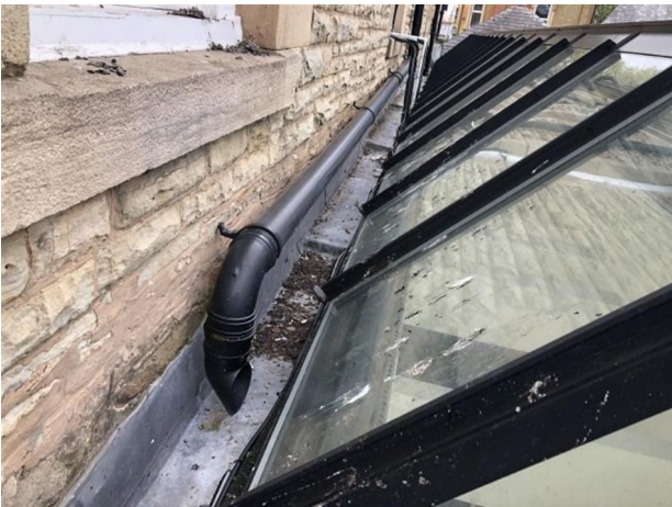
There is a gutter at the back of the structural glazing on roof 1. This is in a good condition and can be left in situ. New 60mm gutters can be formed next to these to take the water to the external chutes.
