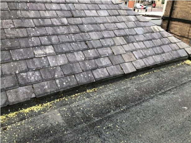
View of the adjacent pitched roof on roof area 1. The lower courses of slate are to be removed to allow the new system to be terminated. The slates are then to be reinstated.
