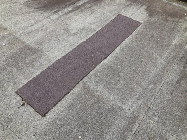
Numerous repairs have been undertaken on both roofs.
