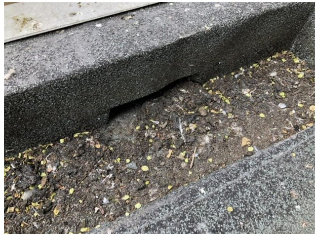
The chutes are narrow on roof 1 and opening these up will rectify this. This will ensure that they do not get blocked.
