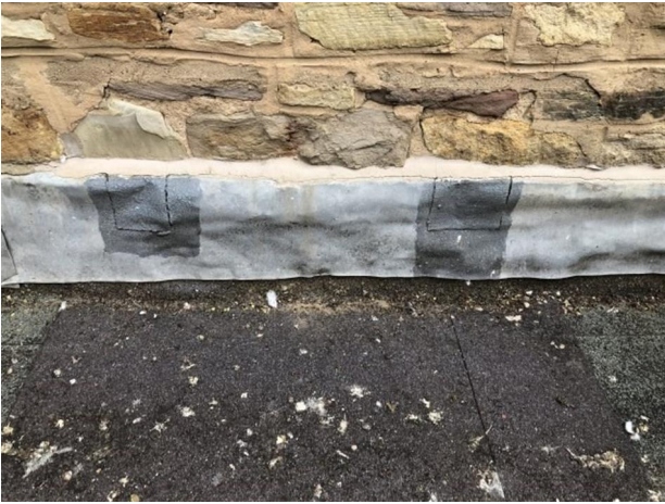
The existing waterproofing on roof area 1 terminates beneath a flashing into the stonework. This will need to be raised to ensure that a height of 150mm is achieved.
