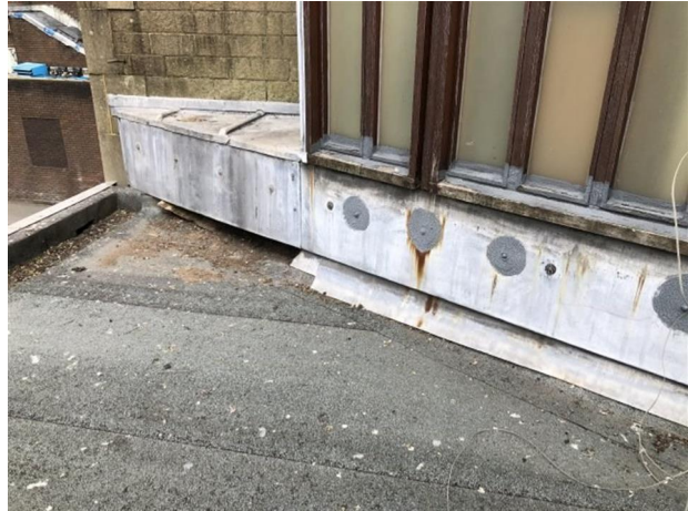
The abutments are to be infilled to level them off and a new flashing installed. A gutter is to be formed on this elevation as highlighted on the roof plan to maximise the height.
