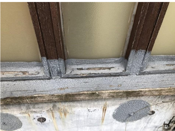
The timber window frames on roof area 1 are in a poor condition. Ideally these should be replaced.
