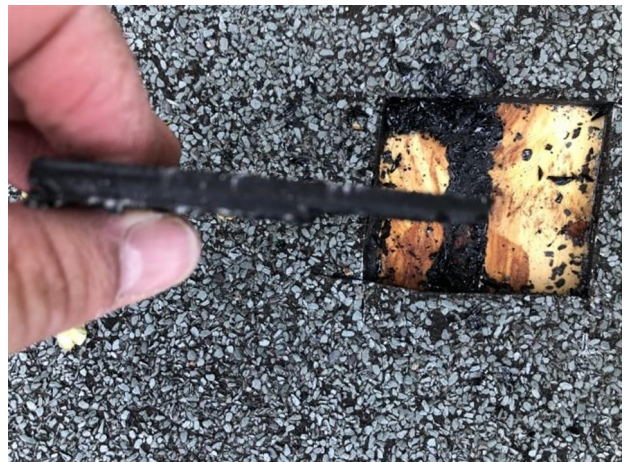
View of the two layers of waterproofing which is beginning to fail.
